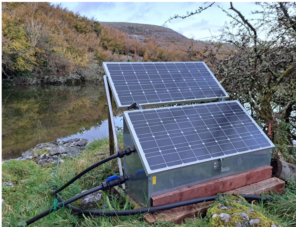
Picture 10: Example of installed Solar Pump
