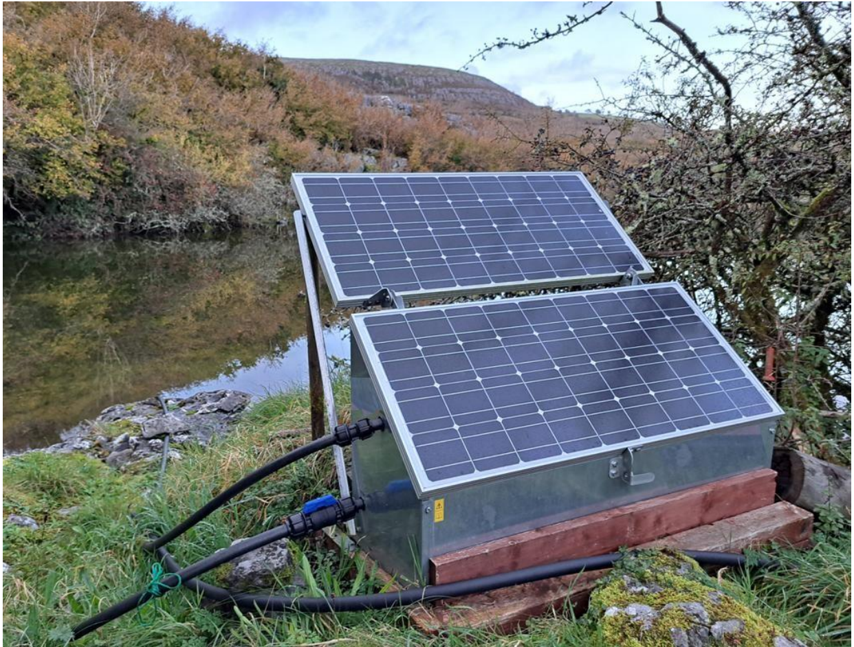
Picture 10: Example of an installed Solar Pump
